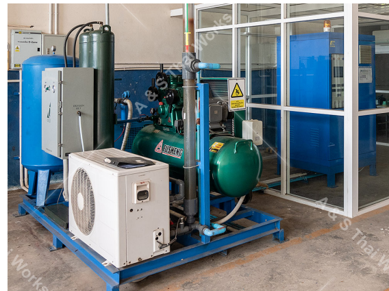
Ozone generating system at fishmeal plant in Thailand
