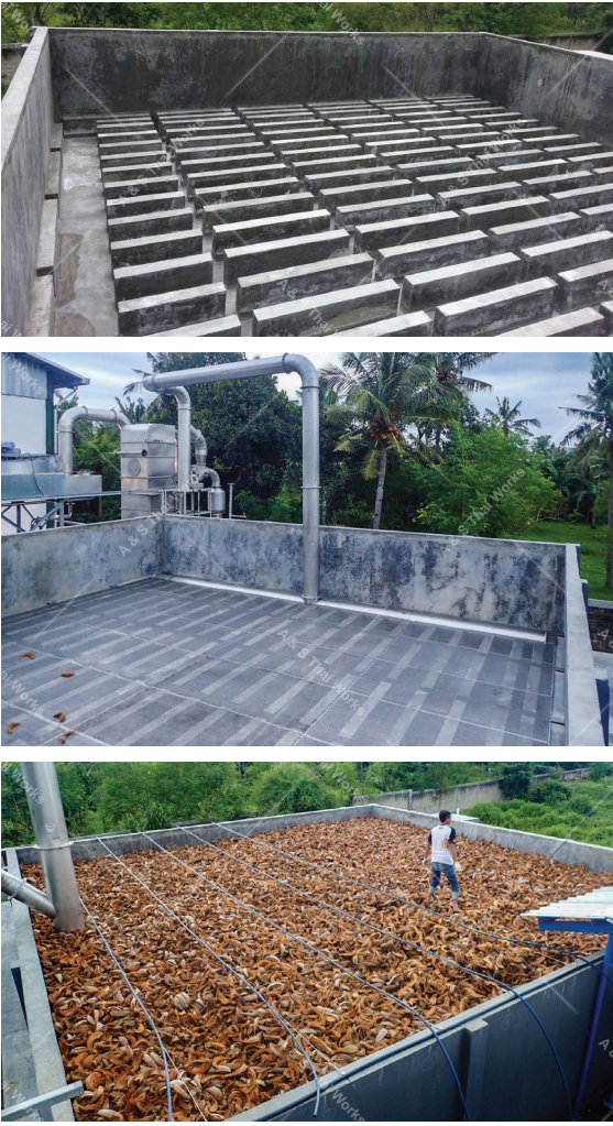
The three photos to the left show three stages of construction of a bio-filter at an ASTW fish meal plant in Indonesia. At this plant, coconut husks are used as “bio media”.
