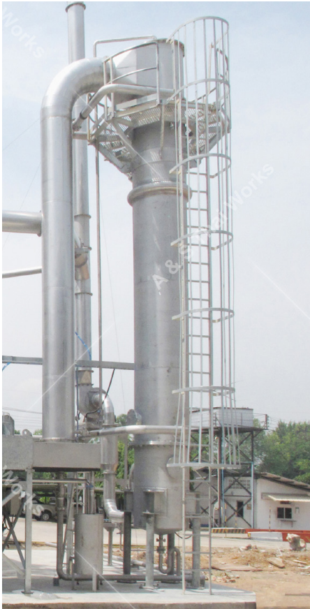
Shell & tube condenser at ASTW fish meal plant in Thailand
