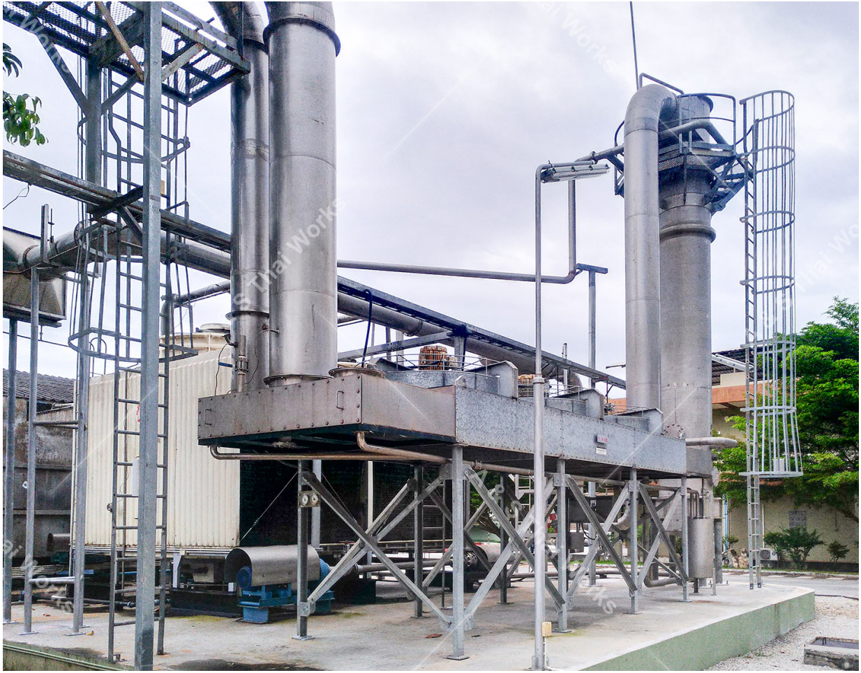
Air-cooled and shell & tube condensers at fishmeal plant in Thailand
